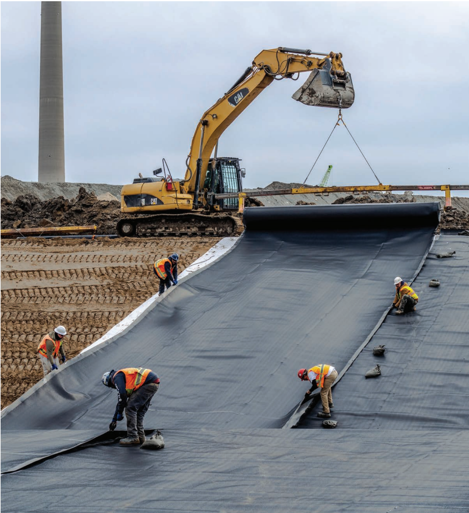
Flood protection work in the Port Lands. Job creation and positive environmental impacts are two key topics in our reporting framework. Image by Vid Ingelevics and Ryan Walker.
