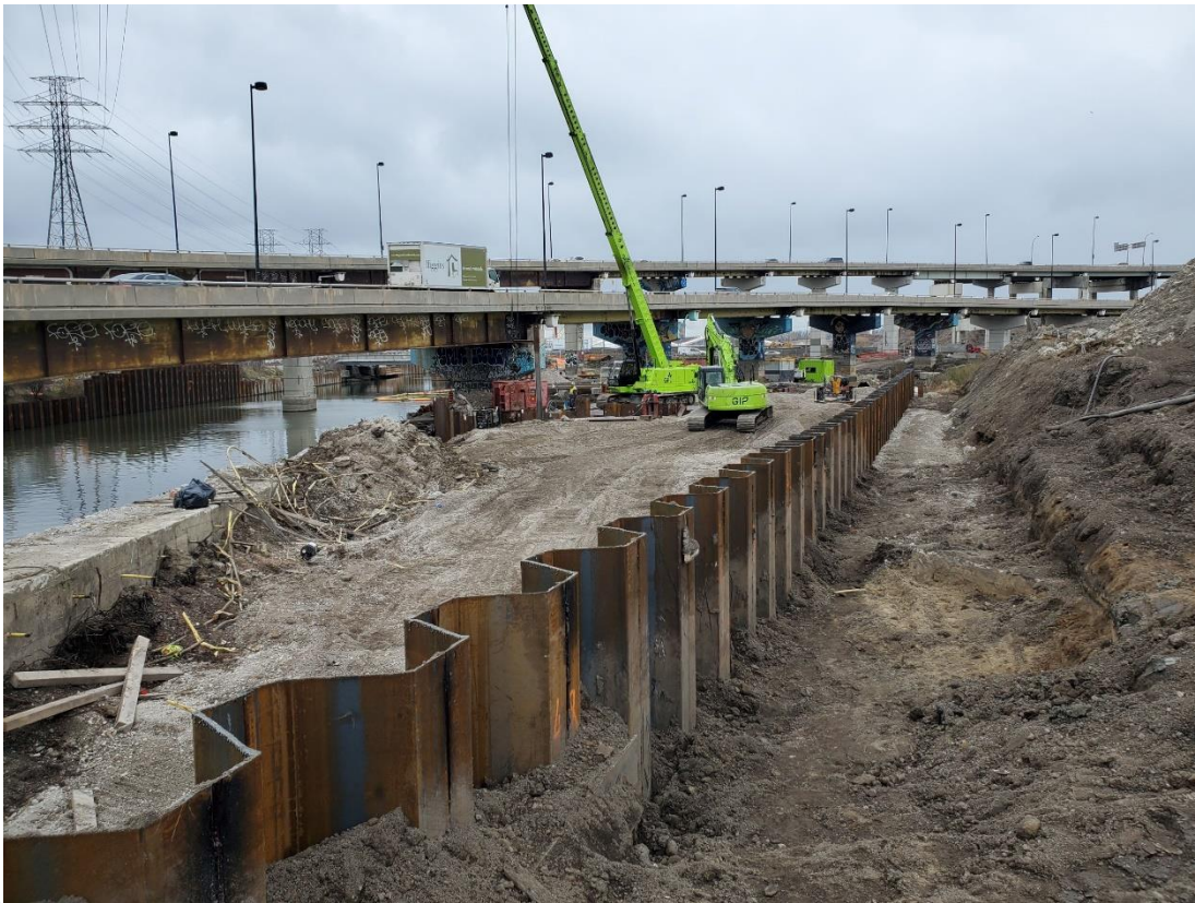
Above: The wall of steel sheet-piles shows where the river will be widened in the Sediment and Debris Management Area. Everything left of the wall will be excavated and become part of the river or a sloped riverbank.
