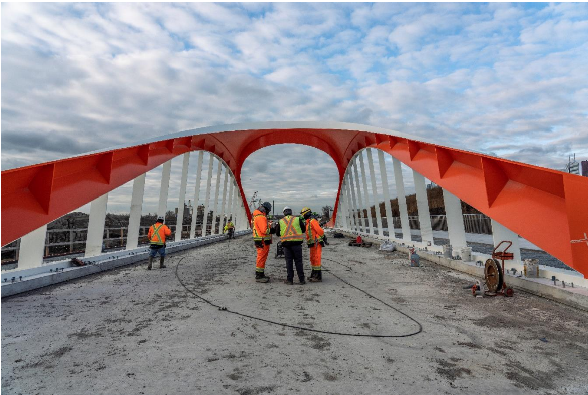
Above: The Commissioners Street Bridge has a deck. The next step is waterproofing and then installing the road base.
