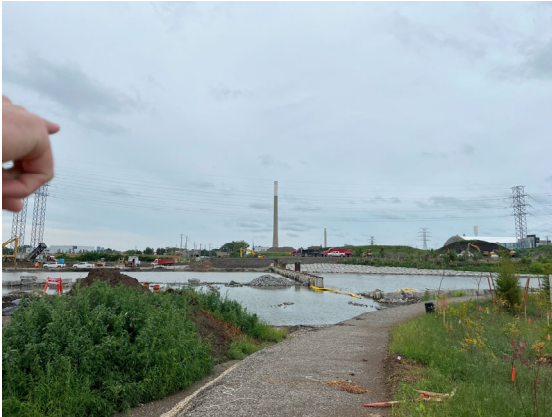
River Channel – River flooded, excavation near the north plug area is ongoing;
