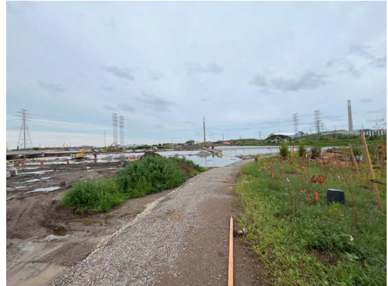
River Channel – River flooded, excavation near the north plug area is ongoing;
