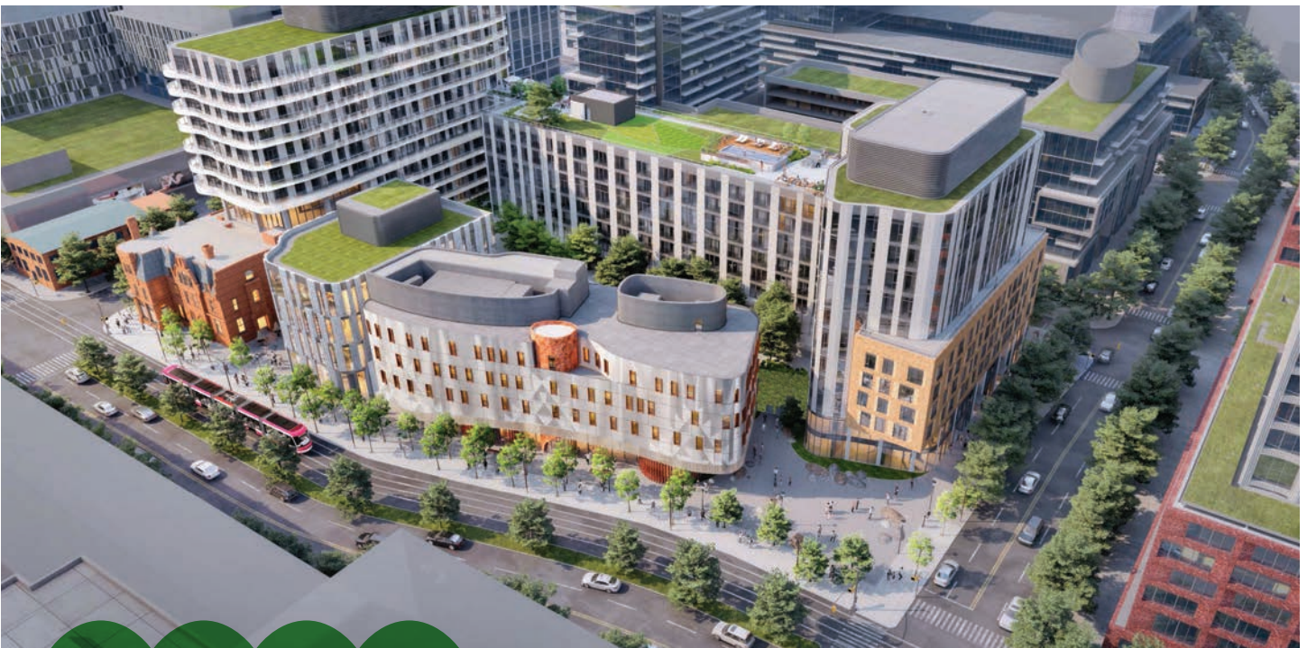
Construction progress continued at the Indigenous Community Hub , a mixed-use development on a city block in the West Don Lands owned by Anishnawbe Health Toronto. The hub will include two buildings (13 and 11 storeys) of condos and rental apartments, as well as a community health centre and a five-storey centre to be operated by Miziwe Biik, an Indigenous-led employment and training organization. Image courtesy of BDP Quadrangle.
