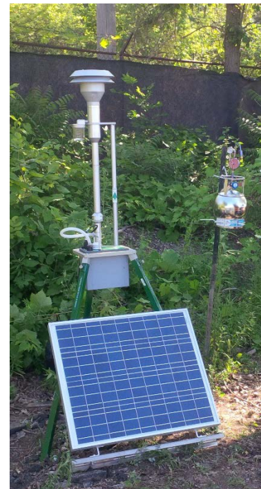
Photo of Typical Air Monitoring Station
