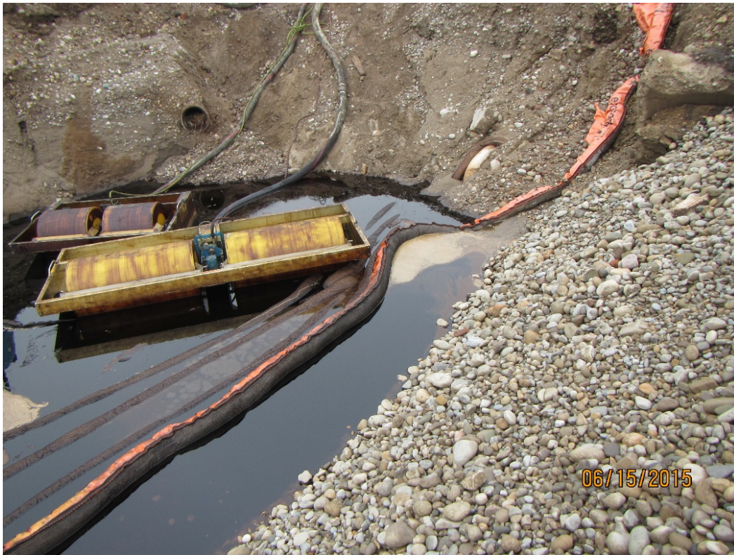
Photo 2. Skimmers Operating to Remove Floating Petroleum Products
