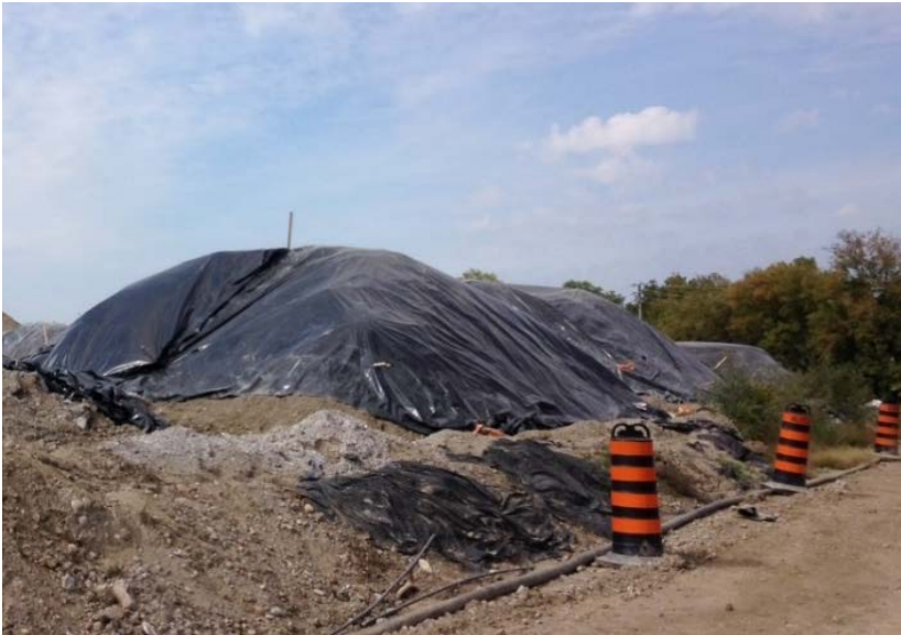
Photo 3. Photo of a Biopile Remediation System
