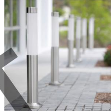
Site-Wide Lit Bollard
