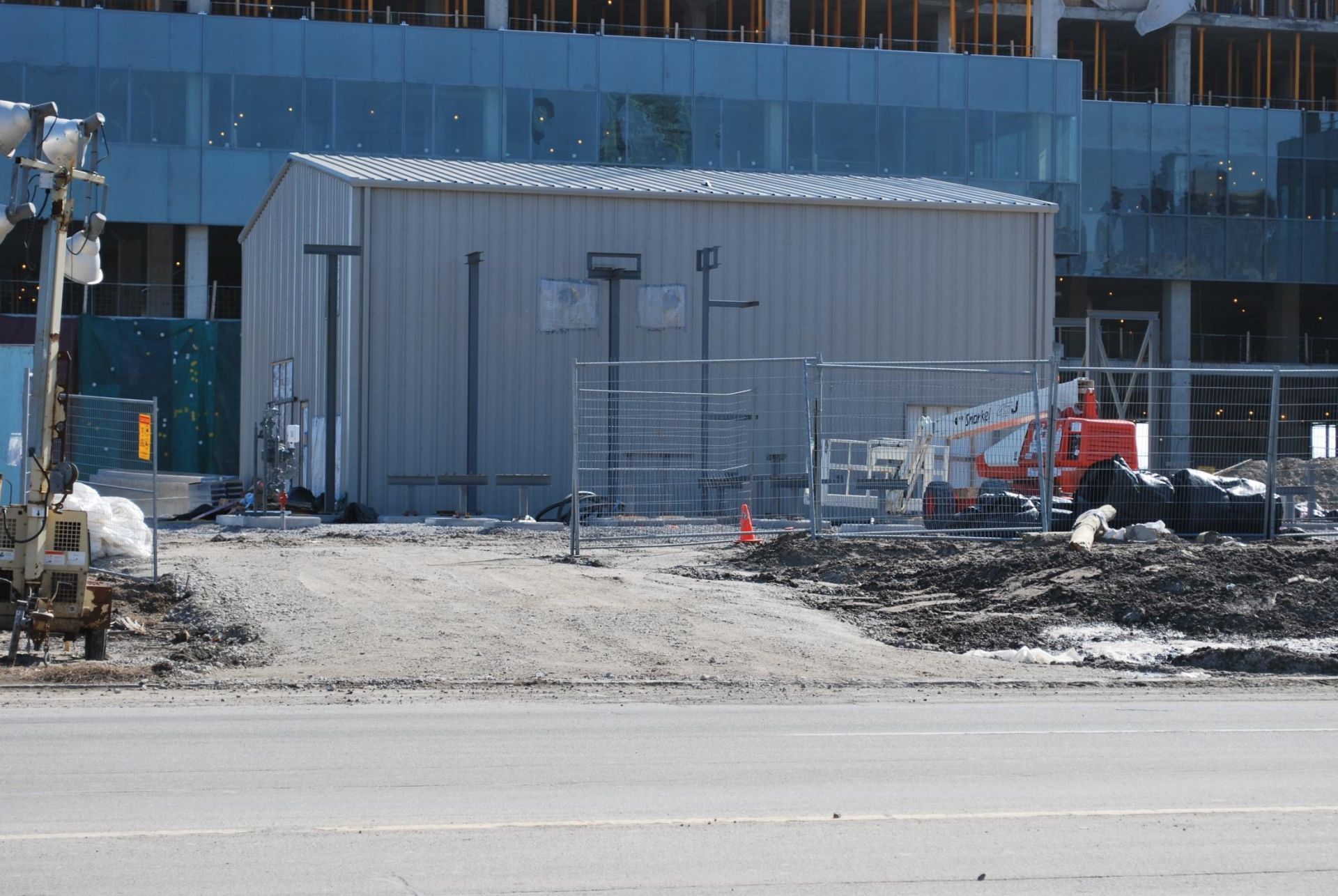
Temporary District Energy Plant Exterior
