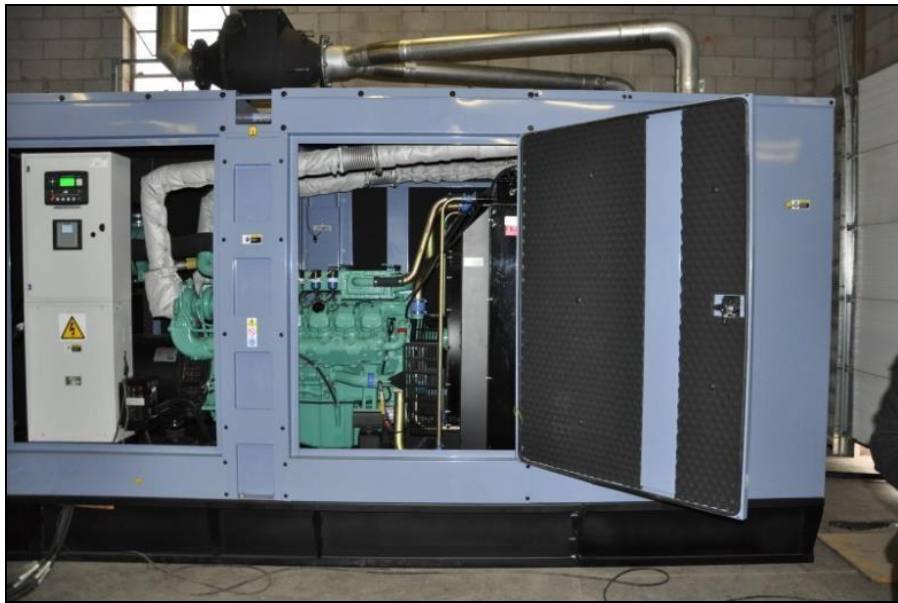
Figure 17. Packaged, 400 kW natural gas-fired generator. Natural gas-fired generators, such as the unit pictured above, are a proven technology that is commercially available. Though more expensive than typical diesel generators, they are more reliable and resilient.
