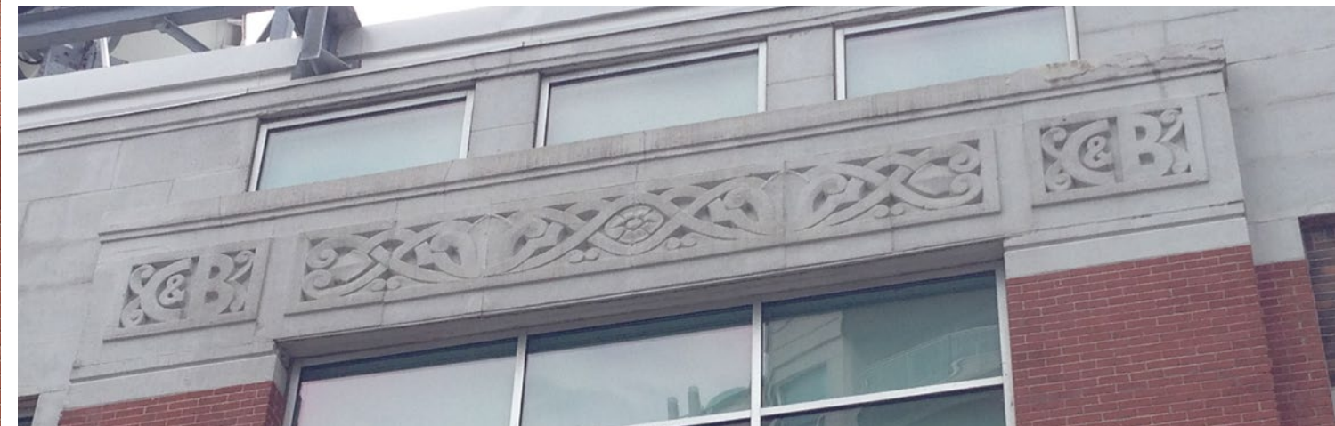
DECORATIVE STONE BANDING WITH CROSSE & BLACKWELL COMPANY LOGO ON THE HEXAGONAL PAVILION & BLDG'S EAST ELEVATION
