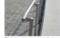
Stainless steel handrail
