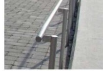
Stainless steel handrail
