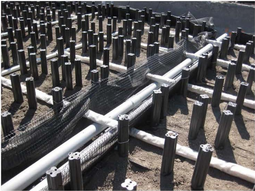
Electrical ducts and irrigation through Silva Cells
